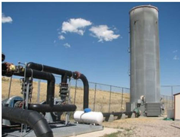
Figure 11 Example of an enclosed LFG flare, from EPA website
